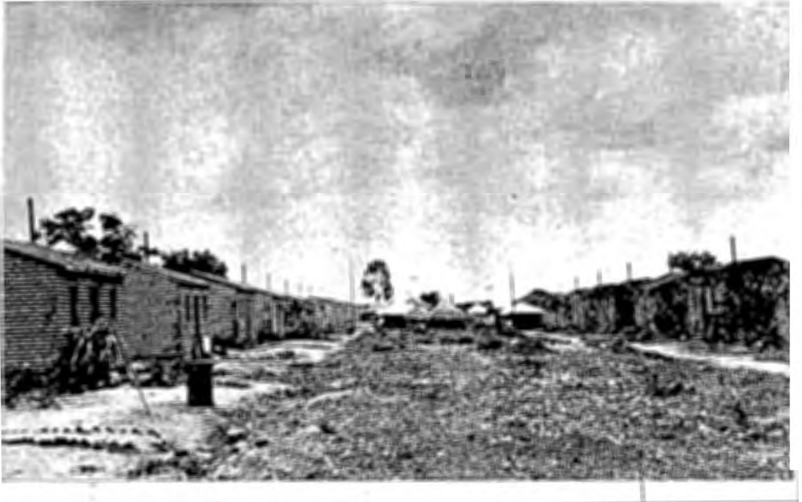
Old huts and shacks being pulled down to make way for new housing: Location 1927.
