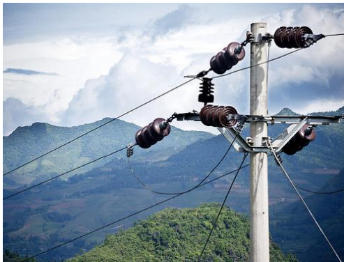
Electrical wires in Bac Ha, Vietnam Photographer: © United Nations by Kibae Park
