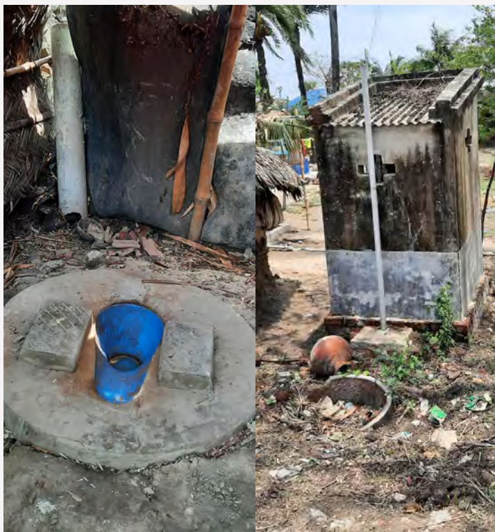
Unimproved WASH facilities at Krishnagar Union, Kaliganj, Satkhira (WaterAid/Md Zarif Oeishik)
