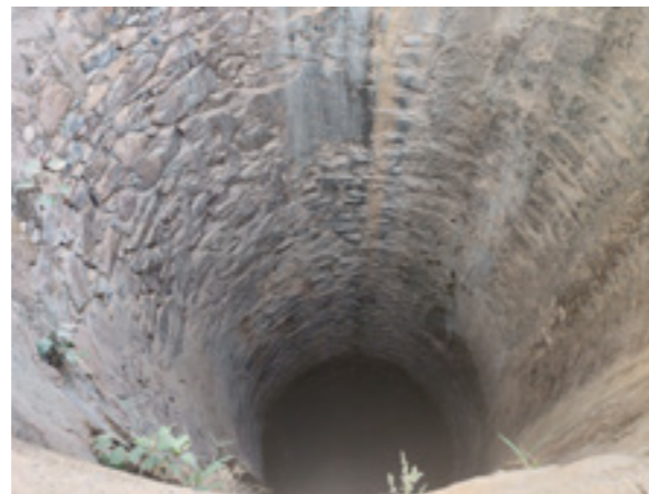
Rainwater collection tanks dry-up and water levels in wells recede during summer in Rajasthan.
