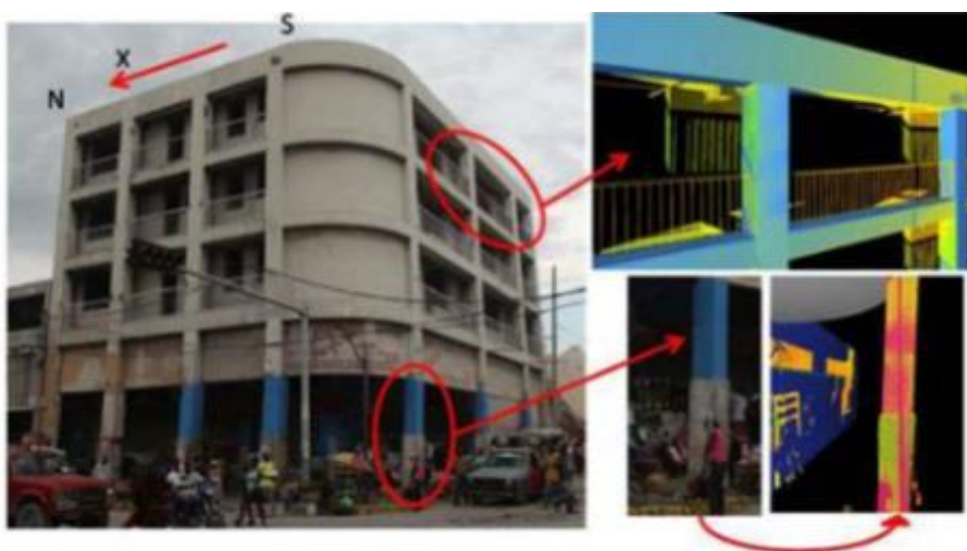
Figure 5: Condition assessment using laser scanning technique, healthy top beams and columns (top right image) and deformed ground columns (bottom right image).
