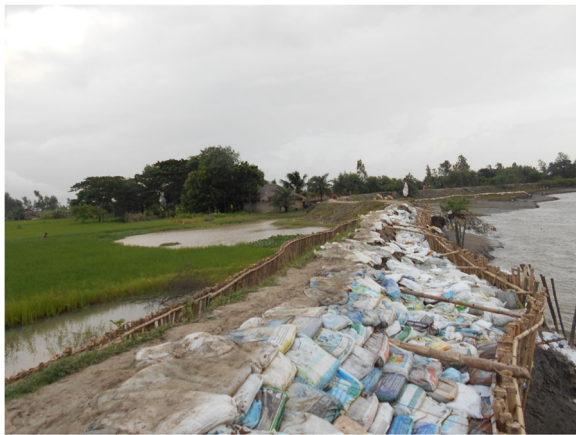
Fig. 7 "All these are the temporary structures of embankment, whereas we need concrete ones. Almost every year our house gets flooded during the monsoon." (Mother 55, age 23, secondary education, fisher woman, general caste)
