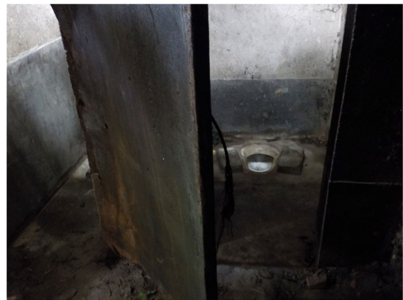
Fig. 3 “In our village primary school the toilet is in a very bad condition – the door is cracked, it is unclean and there is no facility of water. This leads the children to defecate in the open during school time.” (Mother 8, age 30, secondary education, housewife, general caste)
