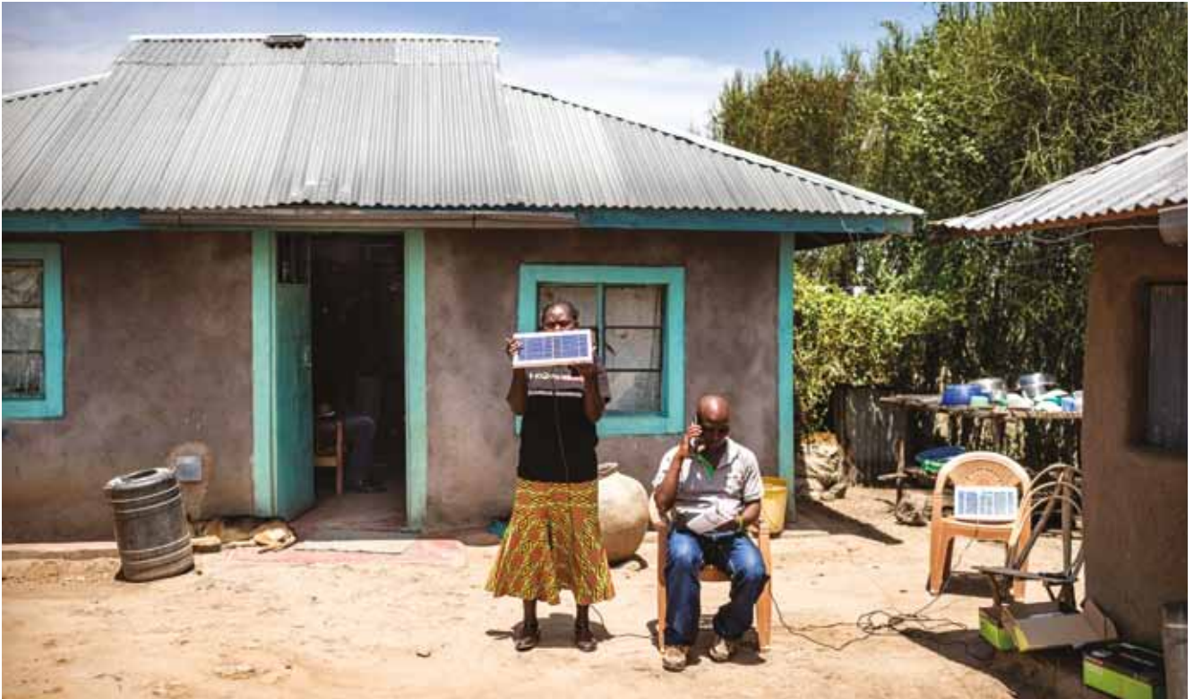
A technician from M-KOPA, a Kenyan based company specialising in low-cost solar lighting, installing and activating a solar lighting system in a rural property. This works thanks to mobile money and sensors connected to the Internet of things. Photo credit: Sven Torfinn – Panos.
