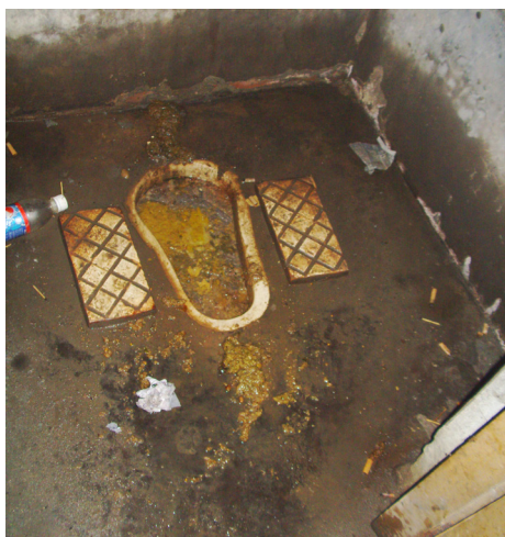
Filled up pit latrine Syedpur Village, Bangladesh. Credit: Suzanne Hanchett.
