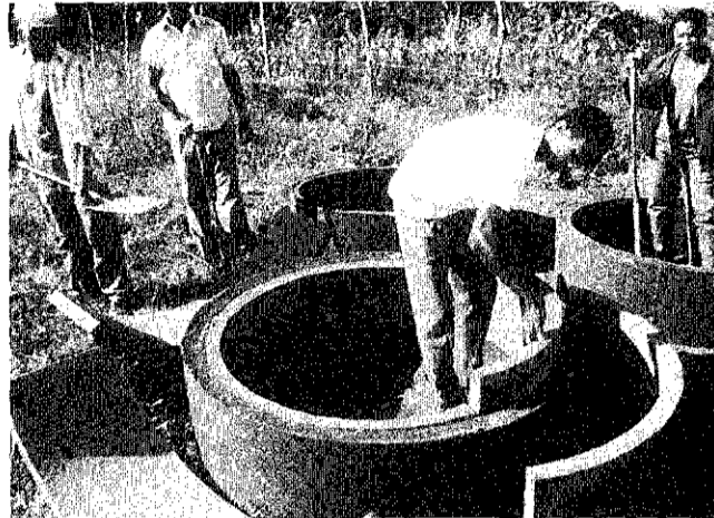
Low-cost water wells are easily constructed by residents using precast concrete rings.
