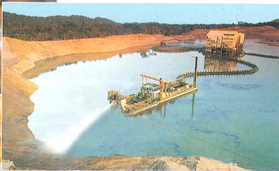
RBM uses a unique dredge mining process to remove valuable minerals from the sand dunes.
