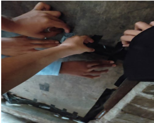
Children repairing the holes in the washroom door. Credit: Nusrat Sharmin © CLARISSA
