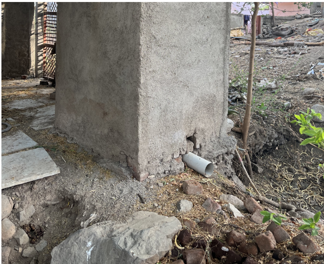
Figure 6: Dysfunctional toilet with outlet not connected to a pit
