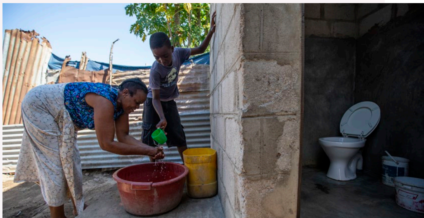
Local residents in Aeroporto B, a densely populated urban area in Maputo Mozambique where Communal Sanitation Blocks have and individual latrines have been installed. (Credit: Jason Florio)
