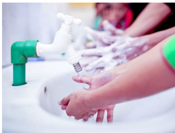
Figure 20: Handwashing at a facility with tap and basin. Credit: UNICEF/UNI310746/Viet Hung (n.d.)
