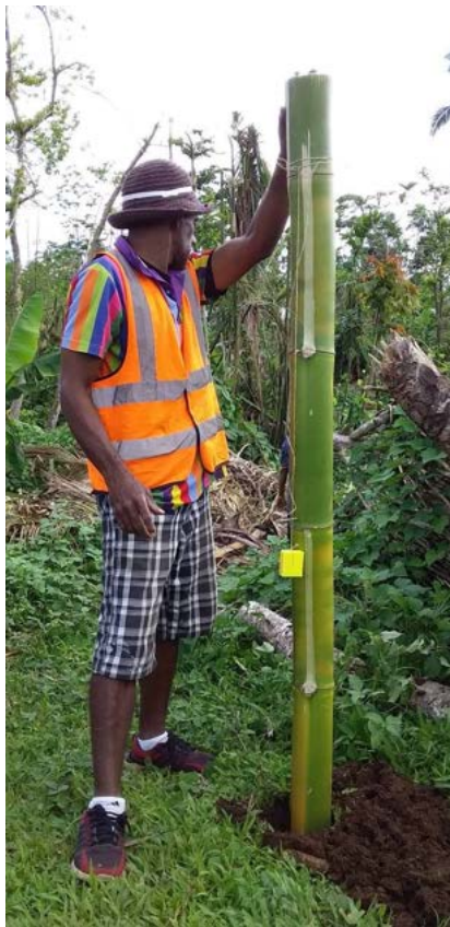
Figure 15: New bamboo handwashing station being inserted into the ground. Credit: World Vision International - Vanuatu
