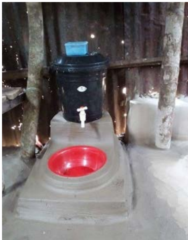
Bucket with tap, installed inside the kitchen along with plastic bowl for basin
