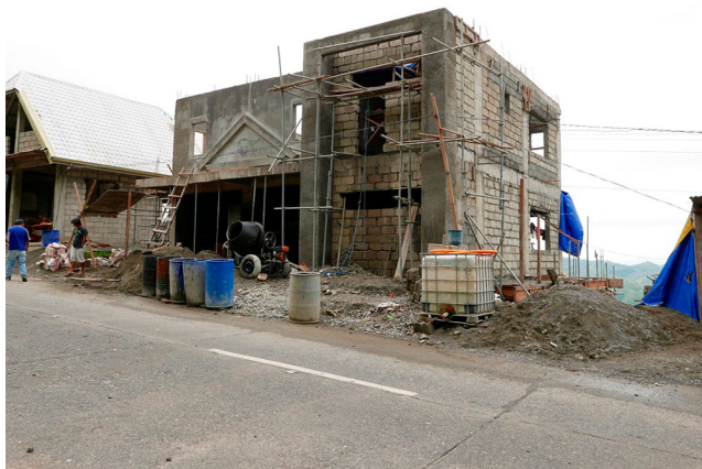
Figure 11. Construction work on new premises for the Rice Terrace Farmers' Cooperative (RTFC), located on the road south of Banaue towards Lagawe. Photo credit: Dominic Glover.
