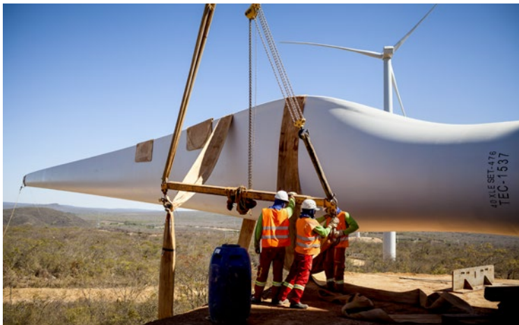
▲ Brazil, Caetite, Bahia State. Workers prepare wind turbine blades to be hoisted onto a new tower in a Renova Energia wind-turbine park.
