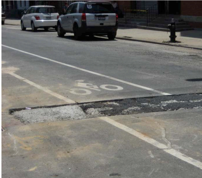
Figure 27: Roadway construction, potholes, utility covers, drain grates and otherwise uneven pavement make cycling on some lanes dangerous. (Source: Lewis Thorwaldson)
