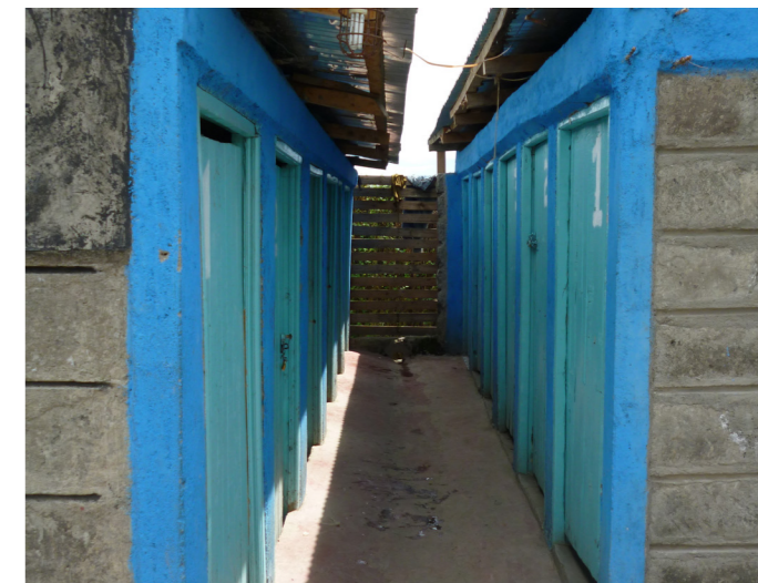
A recently upgraded shared toilet and bathroom facility in Nakuru, Kenya. Credit: Katherine Pasteur
