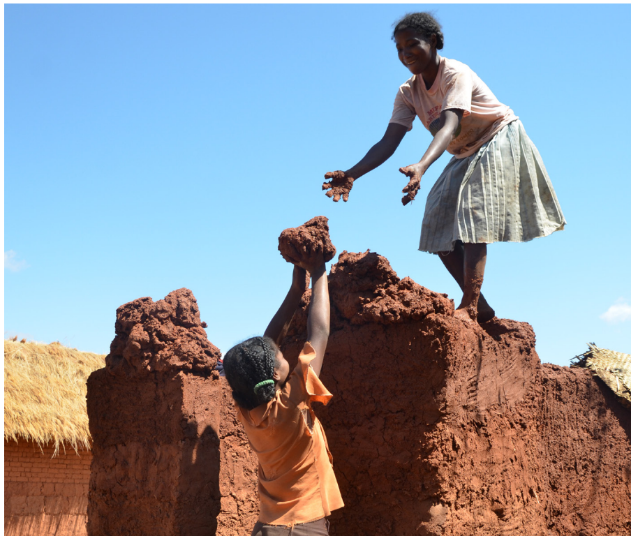
Zinah and her daughter, Zin, 13 years old, building their toilet. Ambohimasina village, Talatan' Angavo commune, Ankazobe district, Analamanga region, Madagascar. October 2013. Credit: WaterAid/ Ernest Randriamalala.
