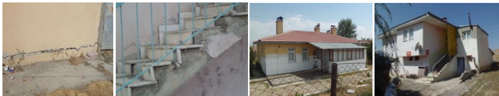
Figure 7 The pictures of the cracks at the bottom of the walls and a sample of the outdoor stair in poor condition with removed top-layer; Additions to the entrances to provide further interior space or storage under the stair (D G Yilmaz 2013).
