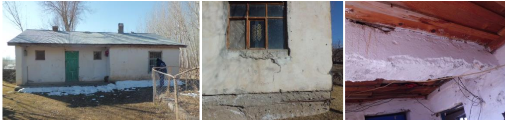
Figure 8 The exterior view of the housing projects for the 1976 earthquake, which are still standing but fairly in poor conditions due to the lack of maintenance; cracks around windows and visible steel reinforcing bars at the bottom of the walls due to plaster loss and an interior beam suffers from loss of section size (D G Yilmaz 2013).
