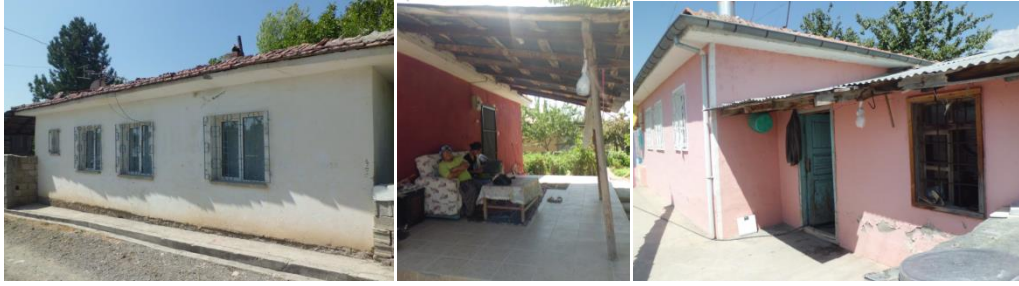
Figure 4 The exterior picture of a maintained house with a facade painted and plastic window profiles; a dweller added a porch to the entrance of the house; another dweller added an extra space to the next of the house (D G Yilmaz 2013).
